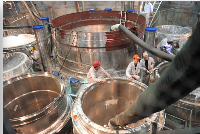
Assembling a reactor in the 'clean area' of the BN-800 power unit at the Beloyarskaya NPP (RIA Novosti / Pavel Lisitsyn)
